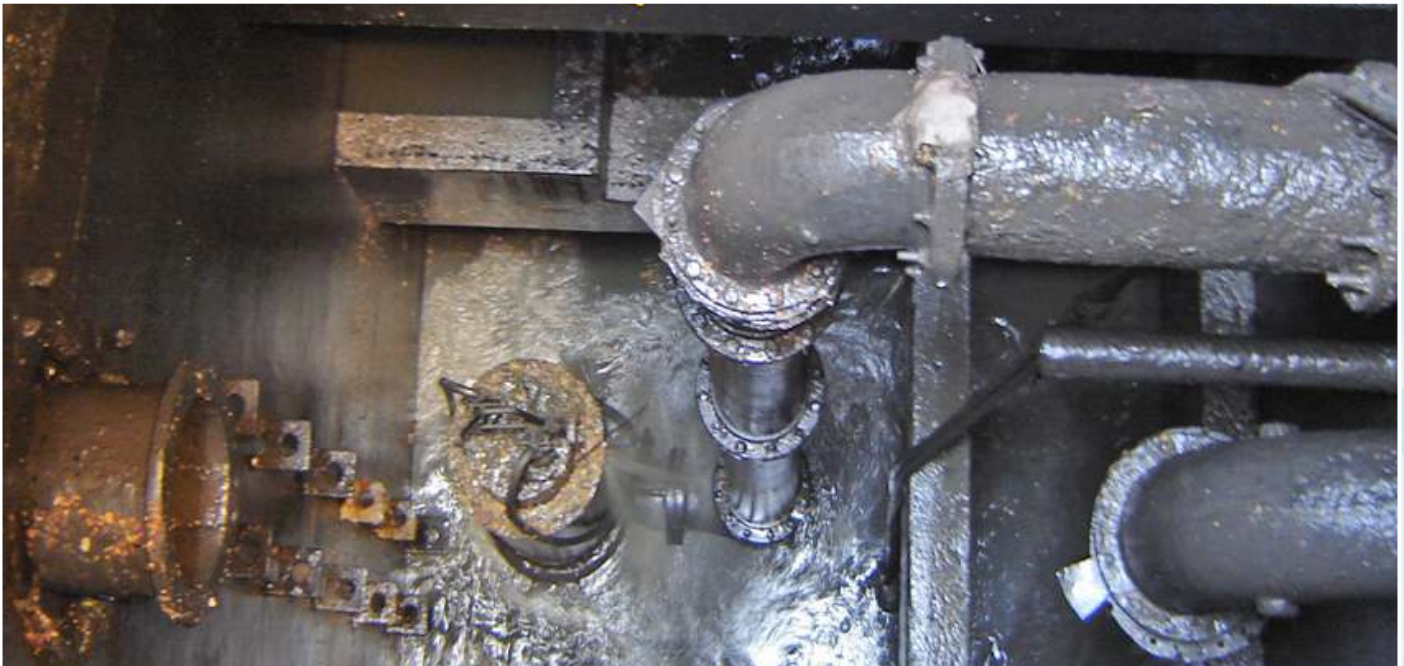
Submersible pump working under very highly turbulent incoming sewage : Salabatpura SPS
