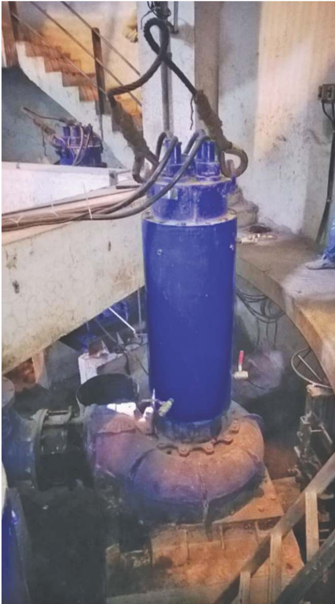
Submersible Flood Proof pumpsets, Navagam SPS
