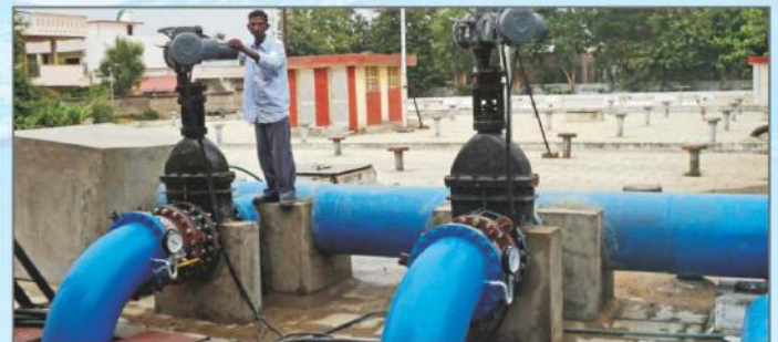
Ahmedabad Nikol Lilanagar WDS 1800m 3 /hr SCF Pumpsets for water distribution directly from UGR
