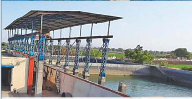
Gujarat Water Grid NC4A Raw Water Transmission Pumping Station ( 600hp x 10 Nos. SCF )
