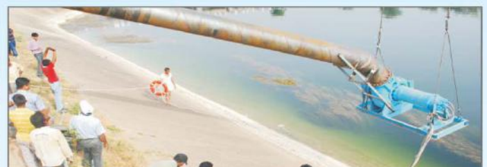
Ahmedabad Jaspur WTP 500mm nozzle SCF used to deliver 150mld directly from canal
