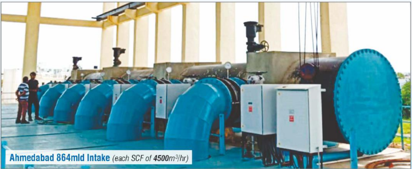
TATA Power Co.'s 108mld Bhira Lifting Station
