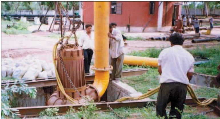
DN 350mm discharge size ANS pump ( weighing 2.5T ) is being lowered for emergency dewatering of a flooded SPS. This pump was run for non stop 300hours in suspended mode without valves.
