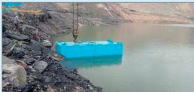
Balasure Alloys Ltd is using 2 Nos. of 250m 3 /hr, 100 m head of 250 HP AQUA Submerged Mine Pumpsets for Kaliyapani Chromite Mines Dewatering.
